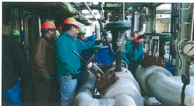
C-Evaps Outage Work-Replacement of a Block Valve and Automatic Control earlier this month.
