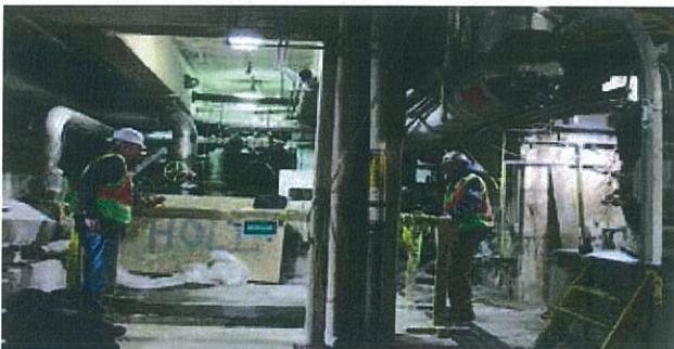
Roberts Company worked with their sub-contractor Concor to prepare foundations for #3 Paper Machine secondary screen and feed pump foundations. Hard barricades were in place with caution tape and signs to alert others that caution should be taken in those areas.
